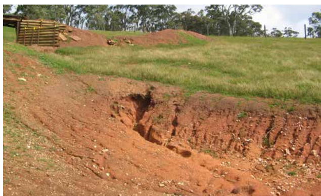
Figure 1: Mass erosion at Upper Hermitage Photo: AMLR NRM Board
