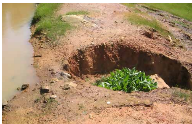
Figure 12: Seepage through the dam wall creates erosion Photo: A. Cole
